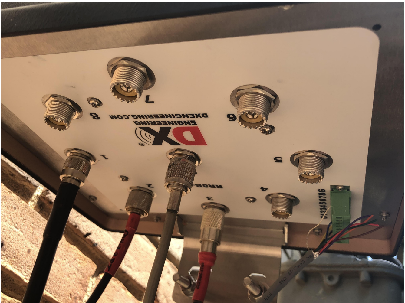
Three connections to the antennas and a center coax sent to the radio. Simple! This switch is a DXE RR8B-HP.
